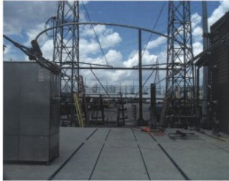
Typical Set-up for Short Circuit Test In High Yard
